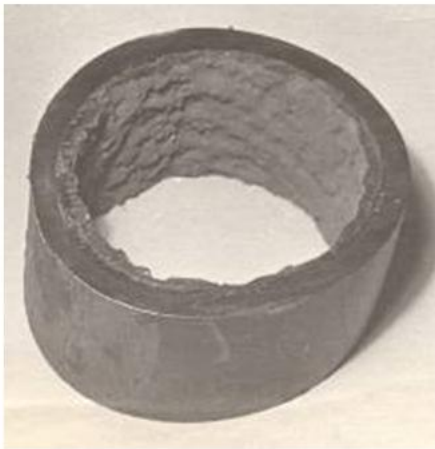
Slag in pipeline
