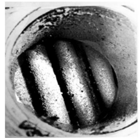
Slag deposit in heat exchanger
